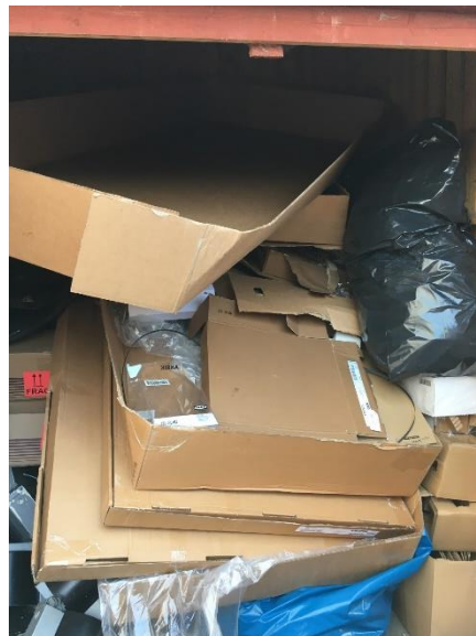
Cardboard pressed into the electric shed. Found during week 34.
